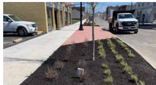
Central Ave., Middletown OH Streetscape revitalization - planting 2000 trees, shrubs, mulching, topsoil and sod installation.
