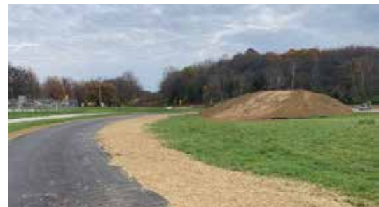
Mount Hope Road Improvements Seeding and strawing, planting trees, and erosion control.
