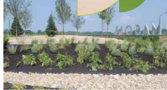
SR 741 Roundabout and Median Topsoil for roundabout & medians Installed 6,000+ trees and shrubs.
